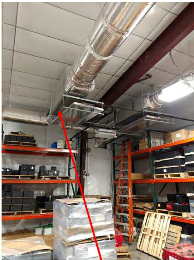
HVAC units located in warm warehouse
