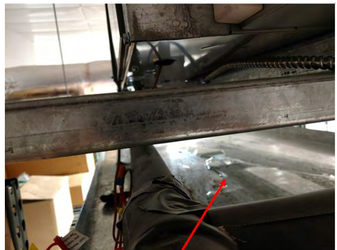
Condensate water in auxiliary drain pan
